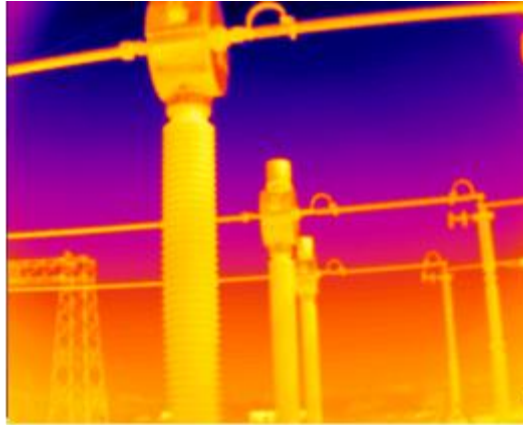
Hot spot in the facilities
