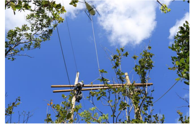
Vegetation too close
