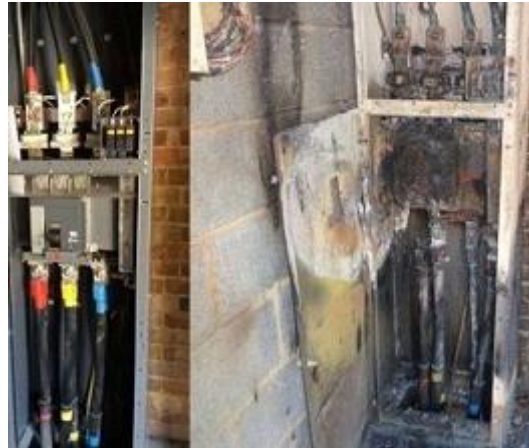
Anomalies in breakers
